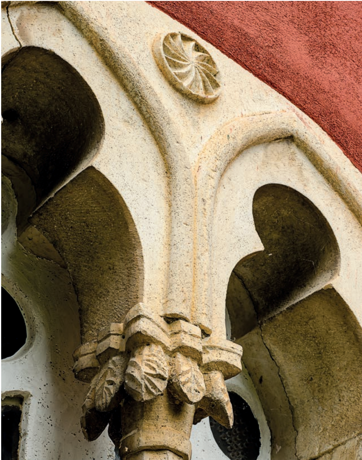
FIG. 171. PEĆ, CHURCH OF THE VIRGIN HODEGETRIA, TWO-LIGHT WINDOW ON THE ALTAR APSE
