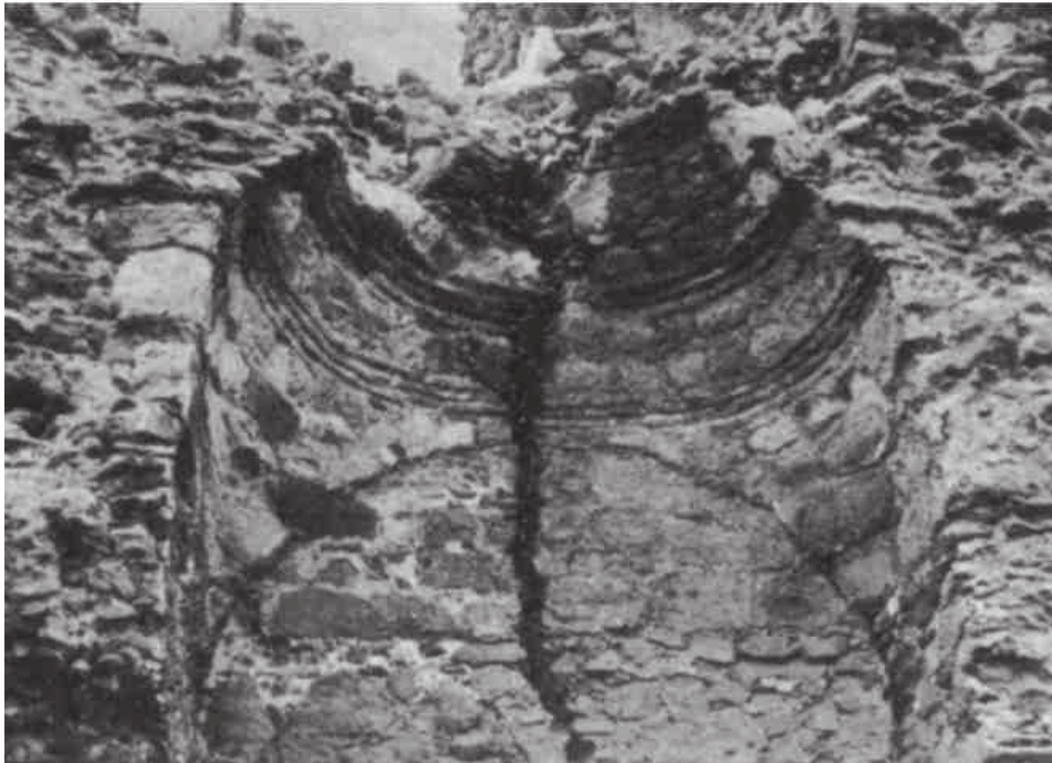
Fig. 4. Smederevo, Fortified Palace; main tower, interior remains before restoration (photo: A. Deroko)
